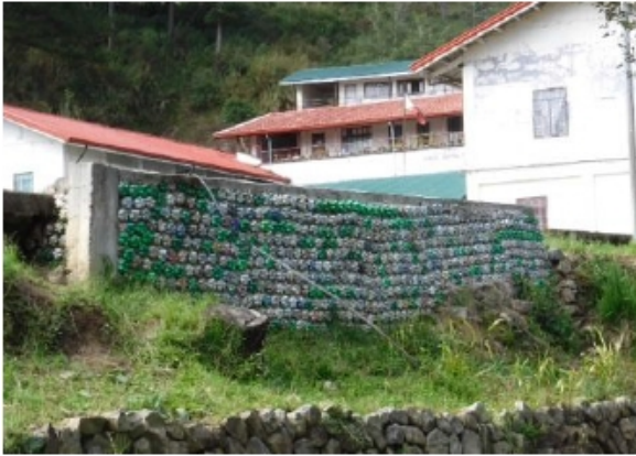
Illustration 17: "Over exposed 'crappy' looking wall"
