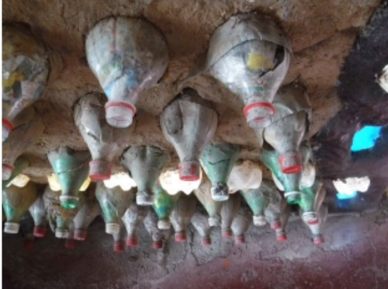
Illustration 5: Bottle tops inside farm house are becoming brittle and breaking. These should have been covered or smaller bottles used.
